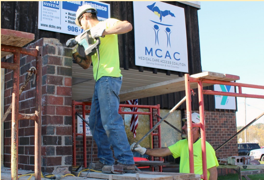
Gundlach-Champion father and son duo Hawkins (left) and Robert Lordson of Perkins remove old bricks from the east side of the Community Center building as part of a job that will see more than 2,000 bricks replaced. The brick work was one of three repair projects that began in October using funds from some of the lead Capital Campaign gifts. The pool mechanical rooms also received attention, and The Markell Company completed its final phase of roof repair.
